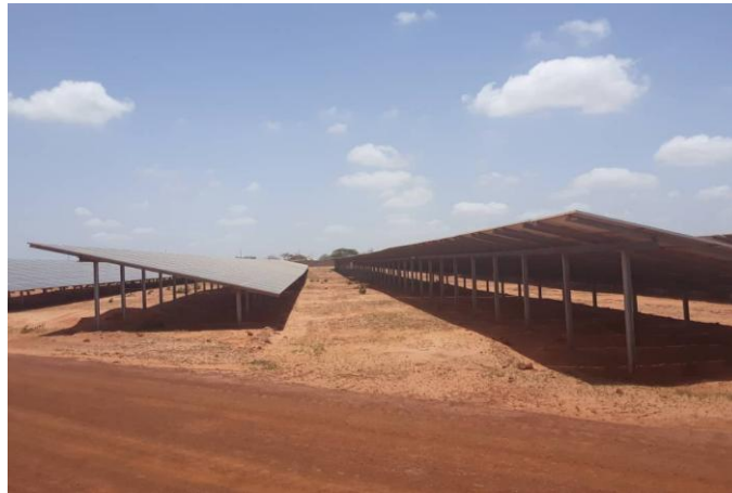
Fig. 1 Diass photovoltaic solar power plant
