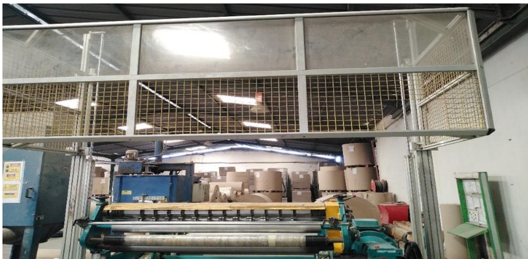
Fig.21 Machine Safety cage
