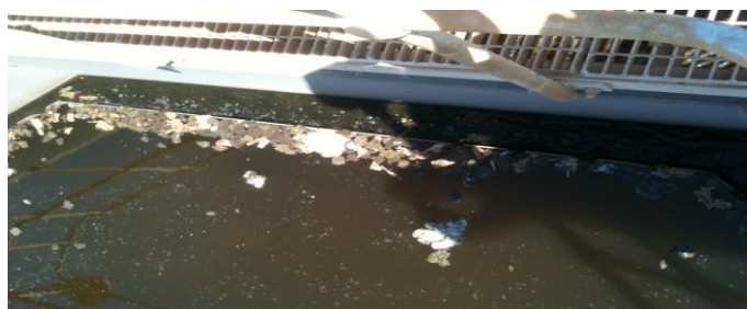
Fig.2 : photo of aeration chamber
