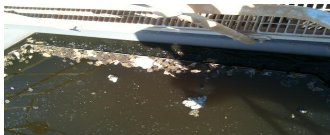
photo of aeration chamber
