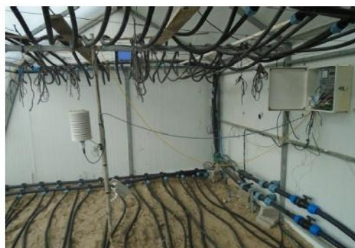
Fig.2. Roof and ground multilayer heat exchangers inside the greenhouse.
